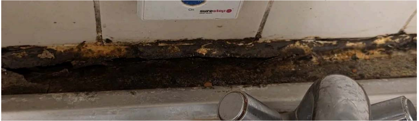
The mould that is currently behind the sink of his home
